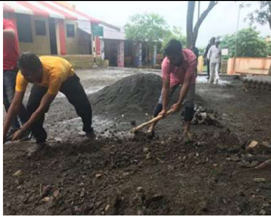
Soak Pit at Tulapur
