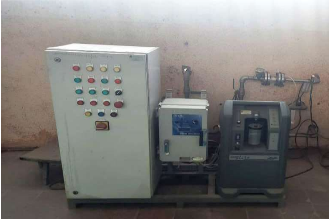
Fig. 2. Actual set up with control unit
